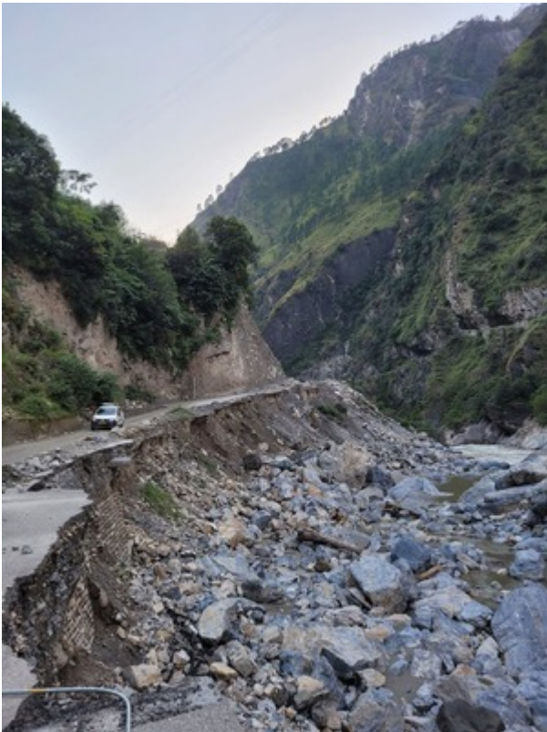
A section of national highway (NH-03) is swept away by flash floods from cloudbursts in the Kullu district of Himachal Pradesh, July 2023. Ashutosh Kumar
